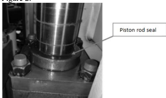
Figure 2 Leakage phenomenon of oil cylinder of opening and closing die
